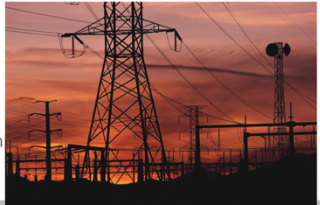
电厂 Power plant
