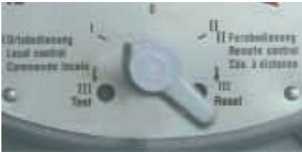
Figure M-3: Selector switch on local controls
